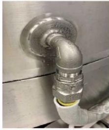
Figure 9 Cooling pipe connection to tank 3
